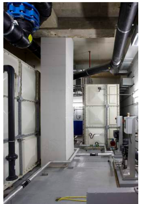
Rainwater Harvesting tanks
