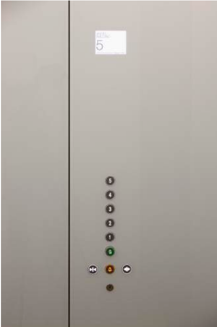
Lift control panel
