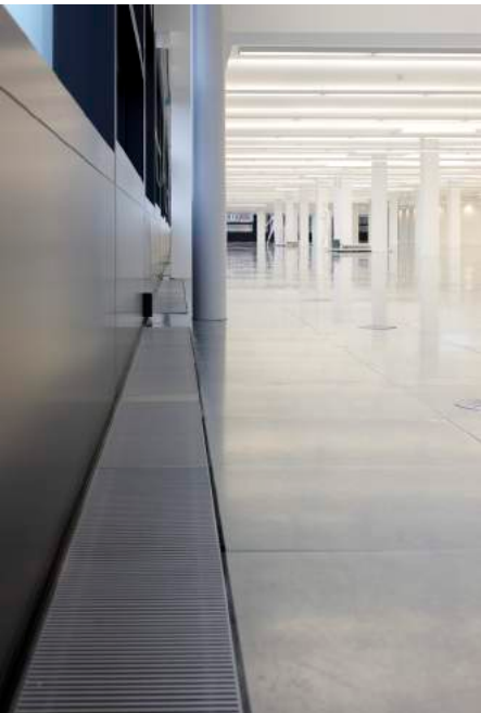
Perimeter heating grille
